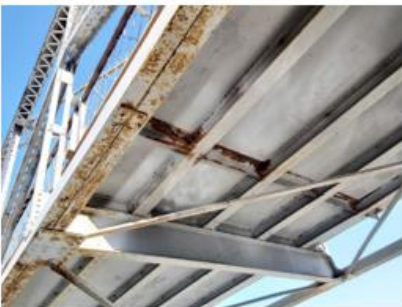
Photo 5: Corrosion on Floor Beam Braces
