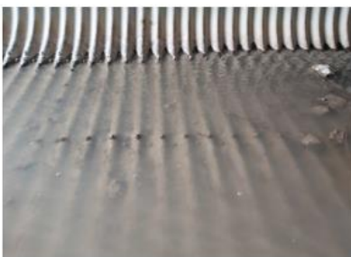
Photo 5: Heaving at Bottom of Culvert
